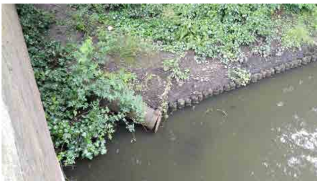
Figure 79 outlet of stormwater sewage pipe
